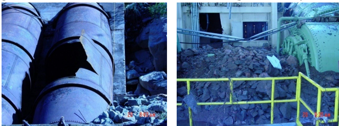
Figure 13: 2007 Shoshone Power Plant Penstock Failure (photos courtesy of PSCo)
